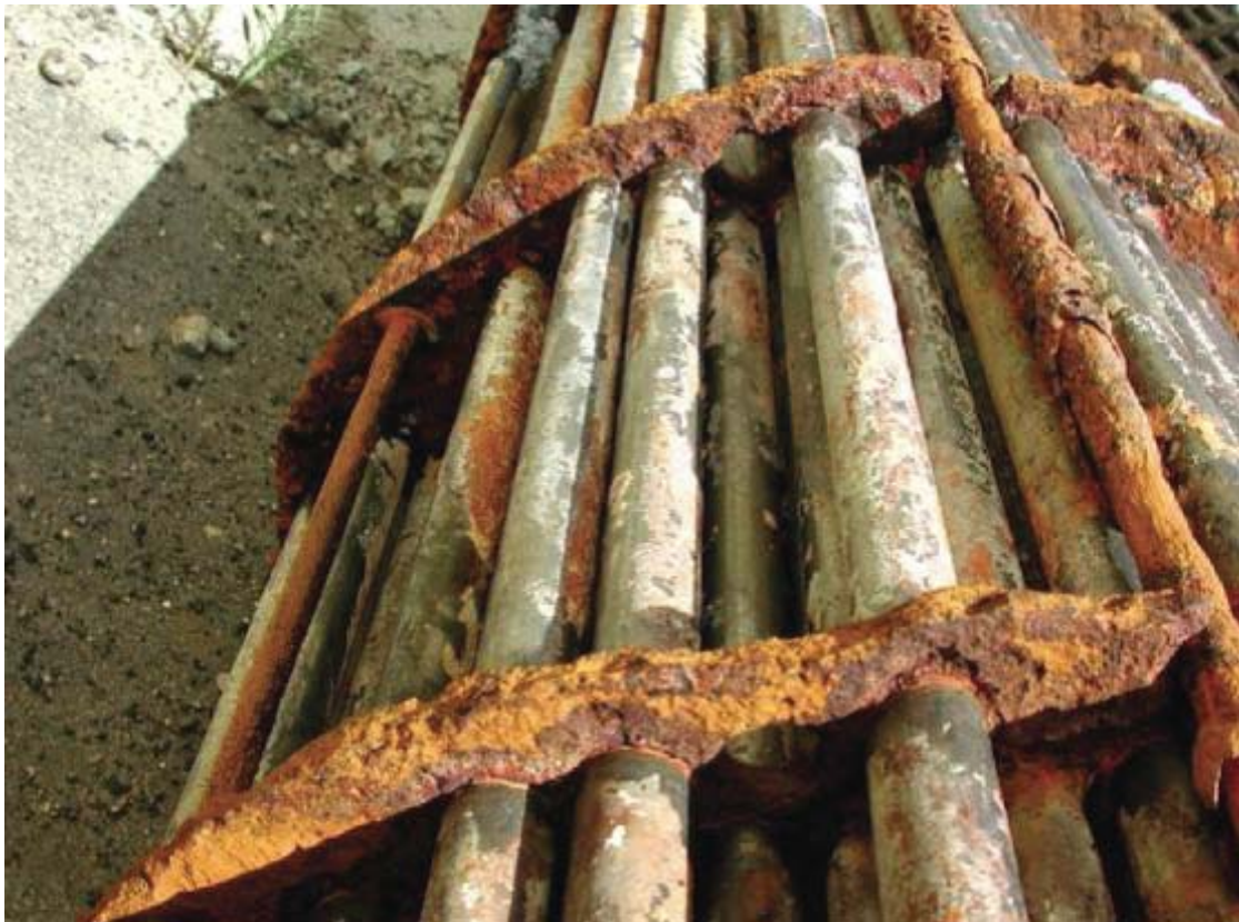
Heat exchanger: tubes made of titanium and baffles made of carbon steel (cooling water, 4 years)
