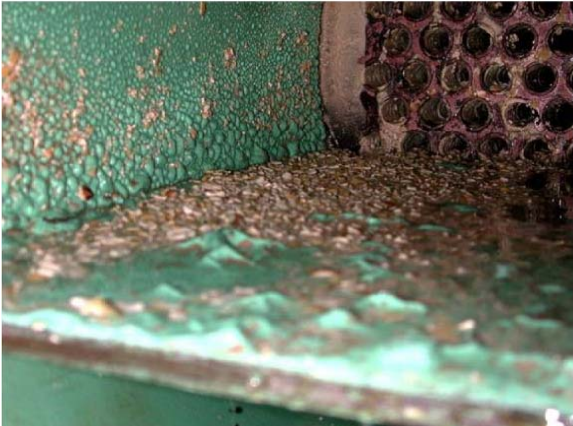
Scale (calcium and magnesium carbonates) formed inside of heat exchanger with cooling water after 4 years
